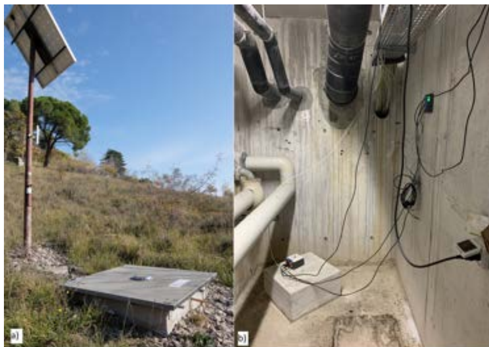
Figure 2. The two typical (a) free-field and (b) inside-buildings installations used in the RAN network. (a) is the the MONF station, while (b) is the POR one.
