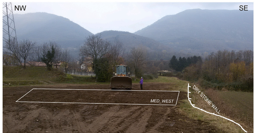
Fig. 16. Paleoseismological trench MED_WEST (a) and relative interpretation (b). Location in Fig. 7. Scarp on the right. One metre for the mesh grid. Note the thickening of Unit 3 toward the South and warping of the contact between Unit 3 and the underlying units in proximity of the scarp. Numbers refer to the stratigraphic units described in the text. Red lines: reverse faults; violet lines: normal extrados shear surfaces. (c) Stereographic projection of thrusts and fractures collected in the damage zone of MED_WEST. Black squares refer to dragging clasts collected on the reverse tectonic surfaces (i.e. maximum stretching of the clasts were considered as a lineation). (d) Spatial relationship between the trench MED_WEST and the scarp: excavation did not affect the scarp, which was strong reworked by human activity. (For interpretation of the references to colour in this figure legend, the reader is referred to the web version of this article.)
