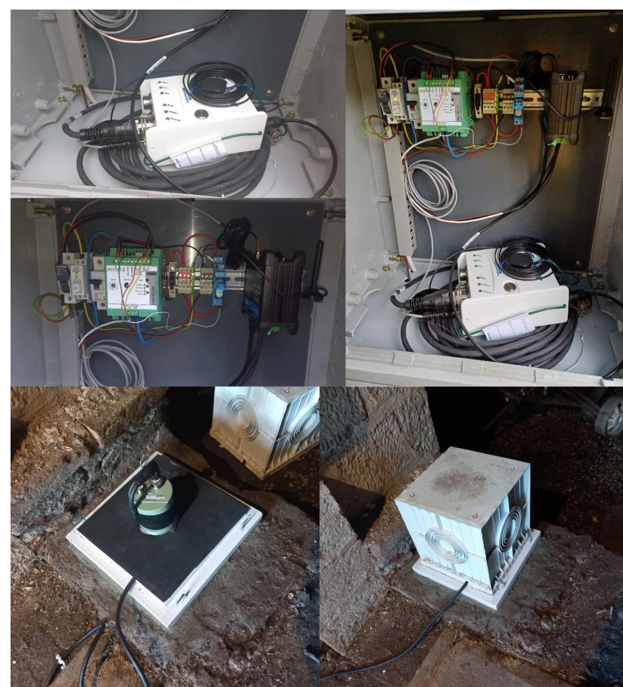
Figure 1. Components of an OGS seismic station for the AdriaArray project (a) the Nanometrics Centaur acquisition system; (b) the mobile internet router with switches; (c) both integrated in a closed metal cabinet; (d) the Nanometrics Trillium Compact 120 sec broadband seismometer, installed on a marble plate; (e) the sensor covered with plastic thermal insulation.
