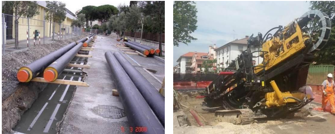
Figure 11. a) Installation of part of the distribution network after the drilling of Grado - 1 borehole. b) Horizontal directional drilling realized under the Grado port canal for the laying of pipeline in 2014.
